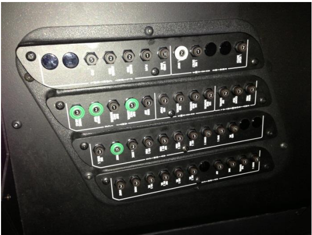
Image 17: Circuit Breaker Panel Pilots Side
