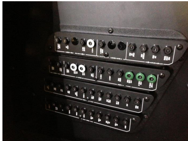
Image 18: Circuit Breaker Panel Co-Pilots Side
